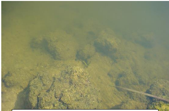
Rip-Rap in a canal, encrusted with small bivalves.
